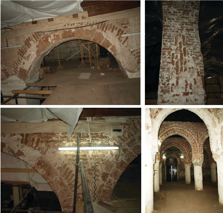
Figure 6: Arcading in the north riwāq – upper left: intact vertical brick lower course and radial brick upper course; upper right: rebuilt arch enclosing remains of the earlier vertical brick soffit; lower left: intact arch to left, rebuilt arch (transition to the present east riwāq) to right; lower right: arcading of the present east riwāq viewed from the north riwāq.
