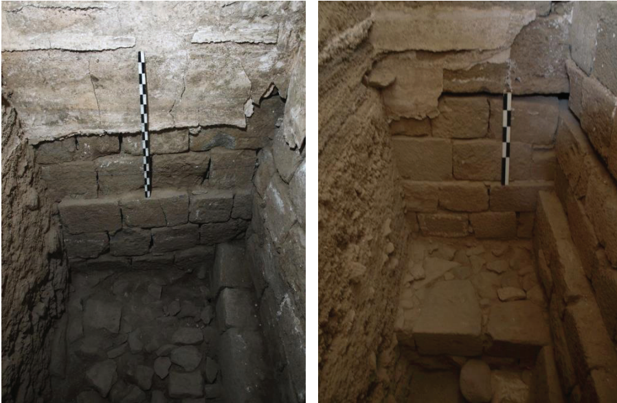
Figure 2: South interior corners of the mosque – left: southwest corner with minaret foundation in center, west wall foundation on right, and wall plaster continuous across the corner (the wood slot is at the top of the partially plastered course of facing blocks); right: the southeast corner after removal of wall plaster, the east wall foundation is in the center and the east minaret foundation is on the right, with the continuous wood slot visible in both foundations; note the bonding of stonework across both corners.
